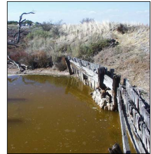
Figure 4. About 60 years ago this levee bank was built to stop the tide coming in to a mangrove swamp so the land could be "reclaimed" for farming or buildings. The mangrove trees all died and the sulfidic sediments dried out. This allowed the pyrite in the sediments to oxidize and form sulfuric acid and rust. The sulfuric acid has killed many of the plants and animals living in this rust coloured water. The acid can also dissolve concrete structures such as pipes and buildings.
