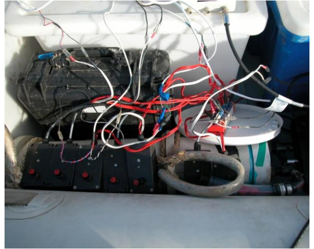
Close up of the pump regulators and bank of 6V, 120Ah sealed lead acid batteries as the power source
