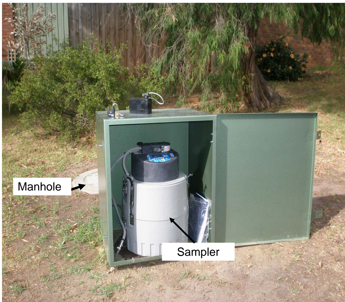
Figure 4: Autosampler installation at site 1
