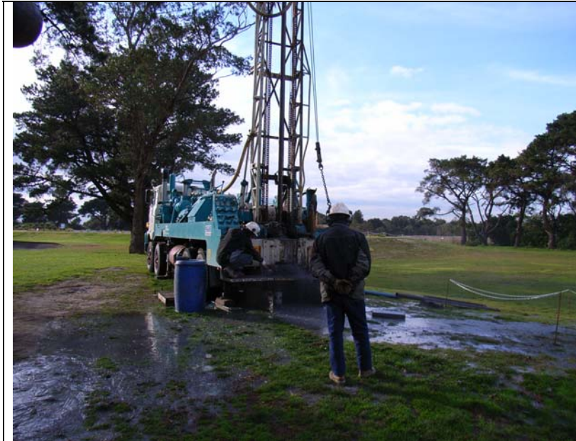
Reaming operations in BH3 performed by Romano Grande (Borewell Pty Ltd) on the morning of 23 June 2006.
