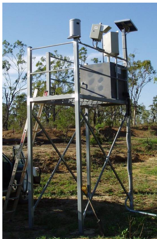
Figure 10. Typical stand for mounting sampling equipment, data loggers, solar panels and rain gauge and telemetry equipment above flood levels
