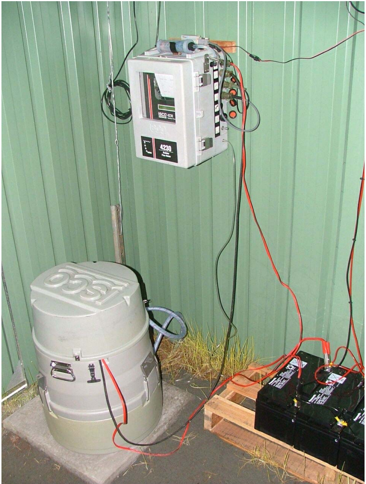
Figure 4. Monitoring equipment at the grapes upper site.
