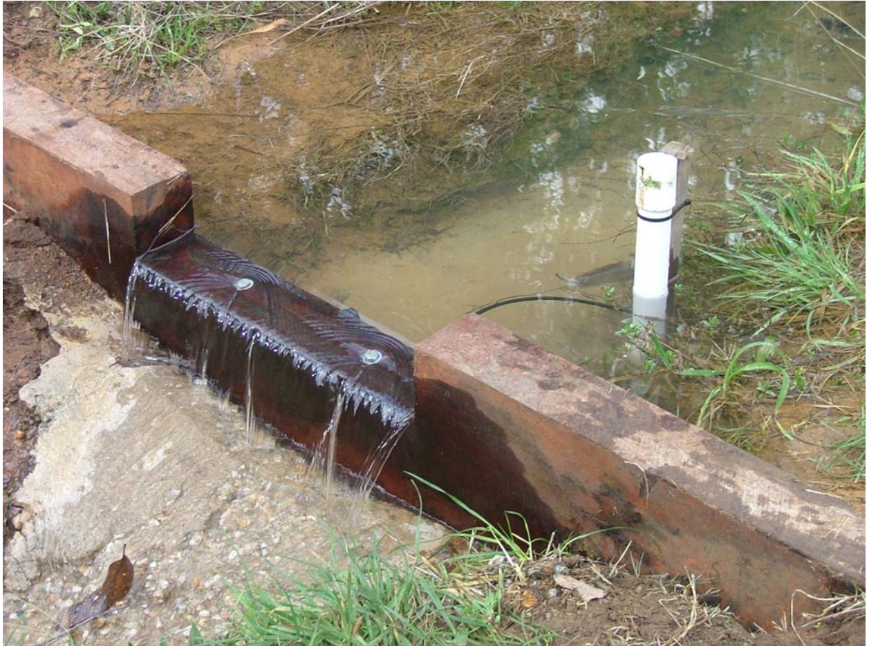
Figure 2. Measurement weir at the cherries site.
