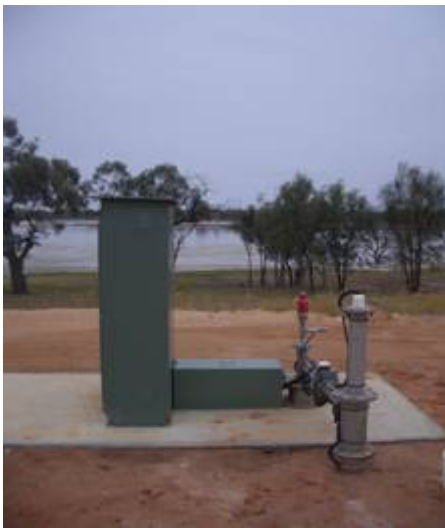
Figure 18. A pumping station designed to intercept saline groundwater flowing into the river and provides an example of captured discharge.
