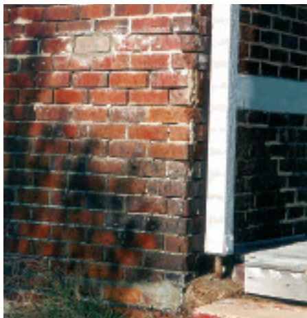
Townsite salinity destroys infrastructure such as roads, public buildings and bridges as well as causing houses to crumble and contaminating water supplies. While often overlooked, townsite salinity is just as serious as farmland salinity.
