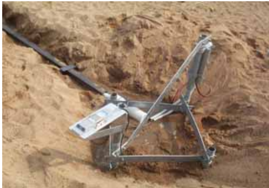
Figure 3.13: Instrument supports in Station Creek
