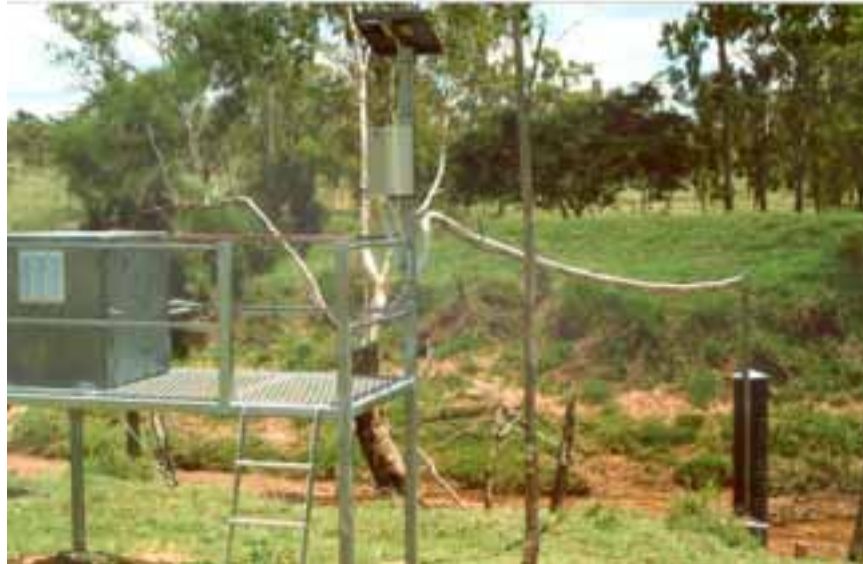
Figure 3.10: Platform at Weany Creek. Box containing auto sampler is on left; datalogger, control unit and solar panel on right hand corner of platform. Sampling device is seen in the background.
