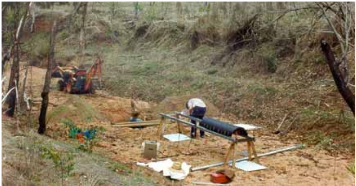
Figure 3.8: Welding poles in place and cleaning out hole in preparation for concreting.
