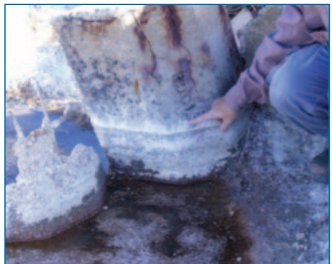
Figure 3a Concrete pipe corroded by action of acid sulfate soils
