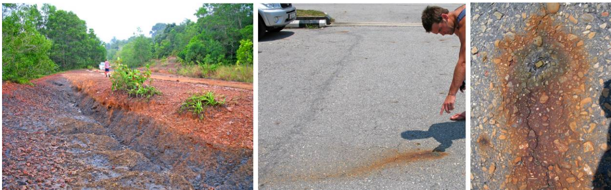
Figure 3. Damage to road infrastructures by erosion and corrosion of concrete and road material (pH 3.5 - 4.2) from the exposure (oxidation) of pyrite contained in the pyrite-rich shale at Tungku.
