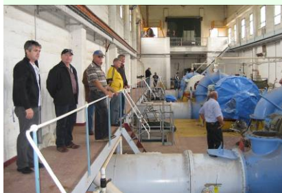
Michael Hoey (2nd left) at the Red Cliffs pump station near Mildura
