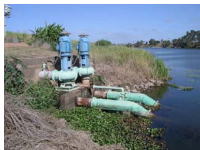
Pump Station at Hutchings Lagoon
