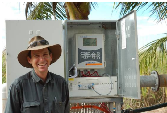
Paul Willis at the computerised irrigation switchboard
